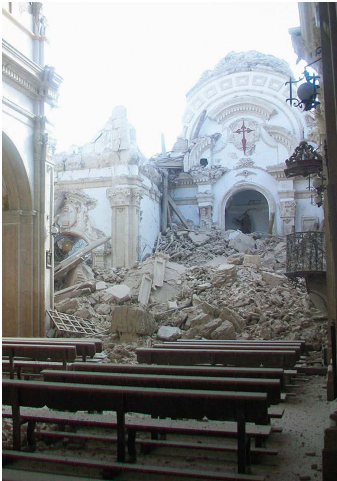
Figure 2- The earthquake in Lorca on May 11, 2011 produced, among other disasters, the collapse of the dome of the church of Santiago.
