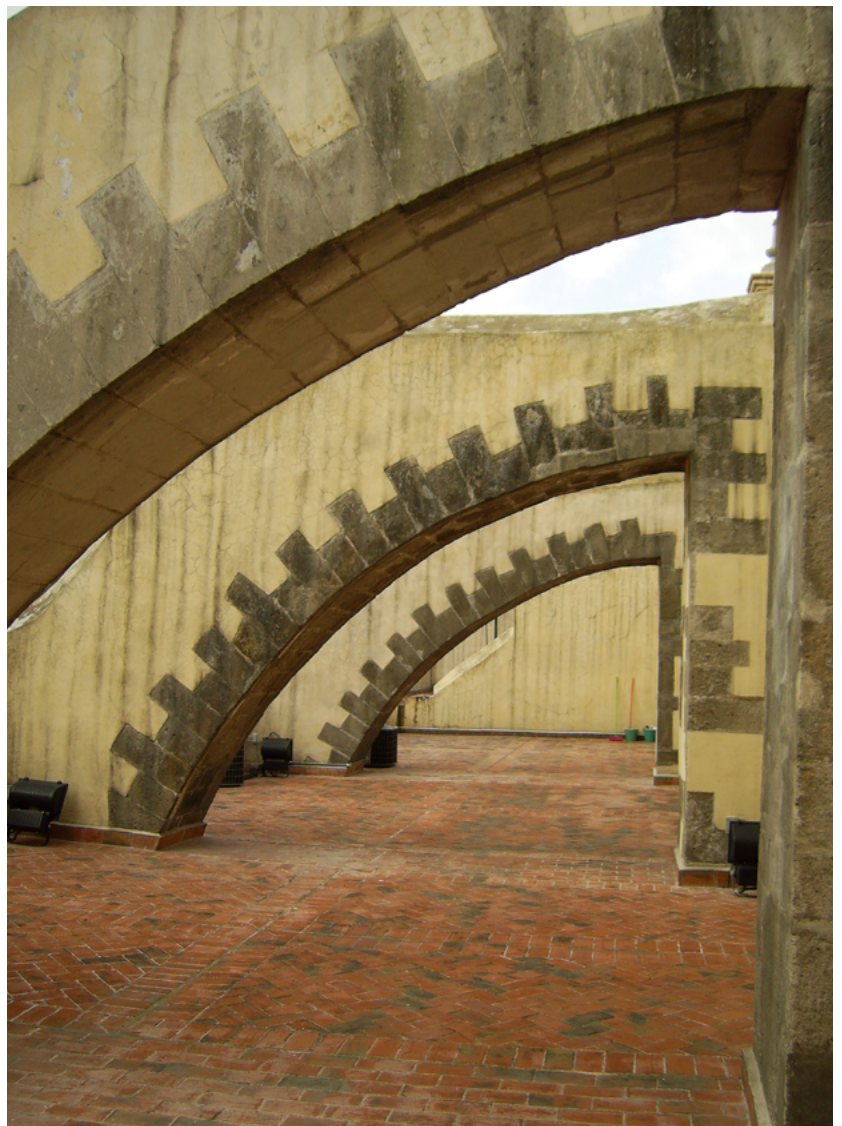
FIGURE 12. Buttresses on the west wall of the vault inserted in 1740, a bad decision made by Fray Juan de Dios de Rivera shortly after Pedro de Arrieta's death (Photograph: Ivan San Martín, April 2019).
