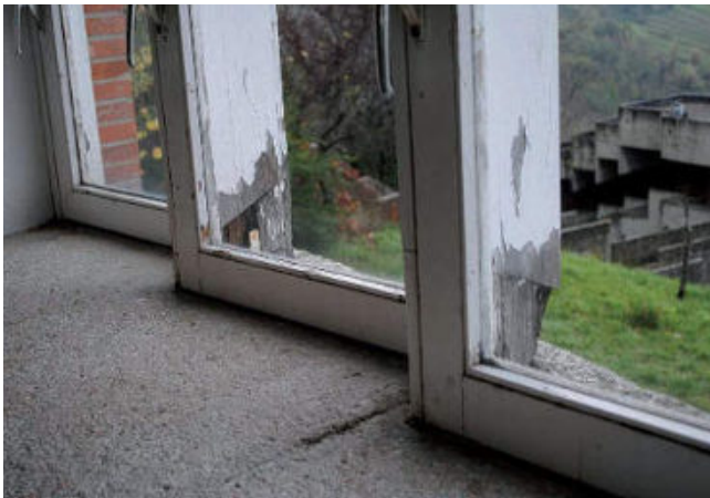
Figure 4.- Collegio del Colle. Decay of the window frames.
