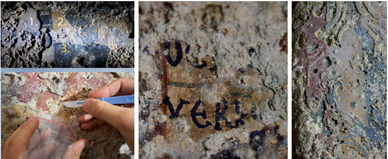
Figure 3.- Photographic details showing the degraded superimposed layers of plaster and the massive crystallization of salts on the painted surface of the wallpaintings; credits: ©Filip A. Petcu.
